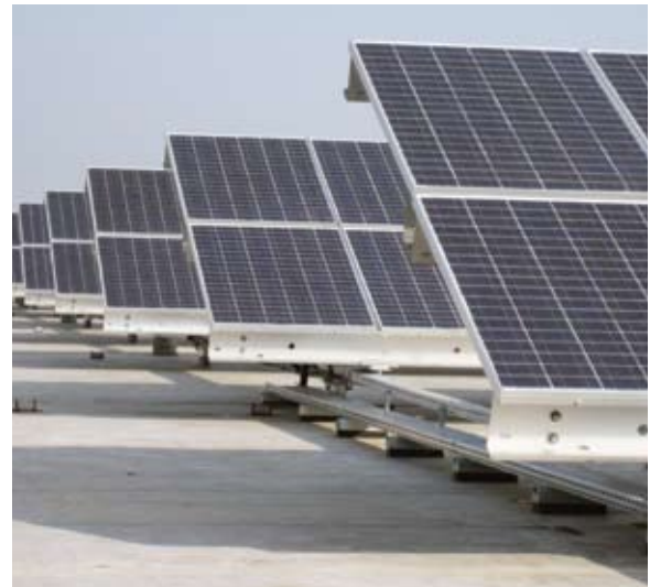
Solar power system installed on the factory roof in Thalheim, Germany
